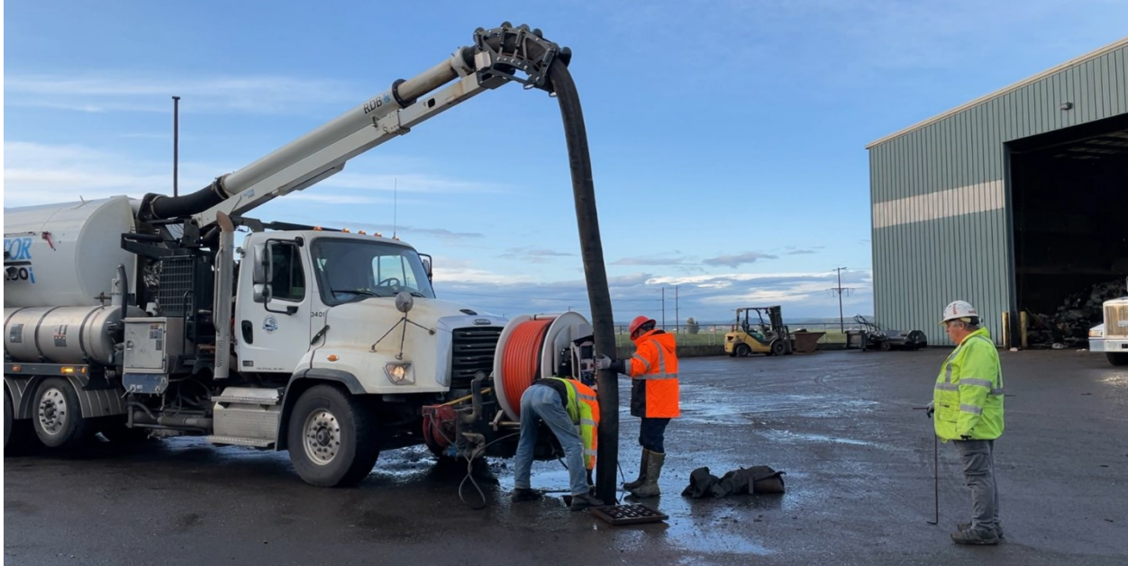
Figure 11-1. A County crew cleans out a catch basin at the Skagit County Transfer Station.
